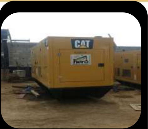
Sound attenuated, weatherproof generator enclosures
