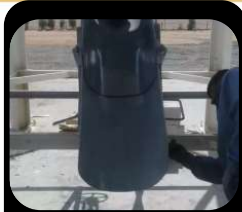
Cement Silos and Related Accessories
